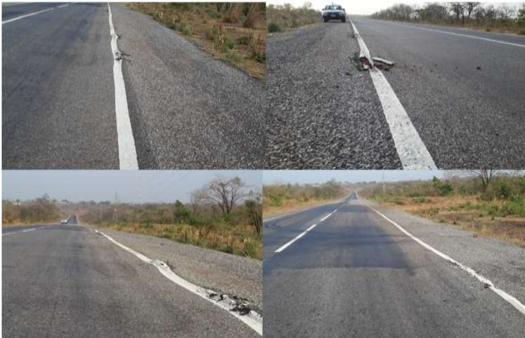
Figure 1. Illustrates some of the defective works executed by the contractor due to poor supervision and the lack of adequate understanding of the contract documents.
