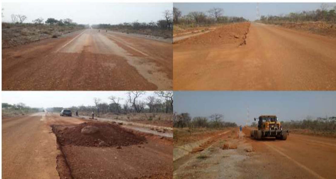
Figure 2. Shows the Contractor's Reworks and defects corrections
